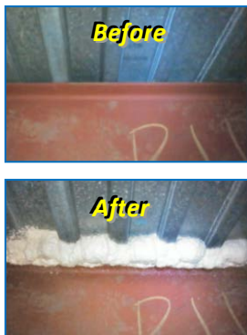
Foam at wall-roof junction
